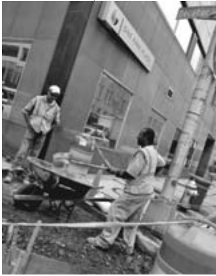
Workers at the corner of Decatur Street and Park Place begin the first phase of construction to improve pedestrian movement along Decatur Street.
